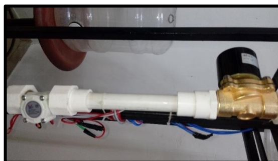
FIG. 6. SOLENOID VALVE AND FLOW SENSOR
