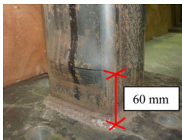
(a) Deformation of NCFHS-0 (left face)
