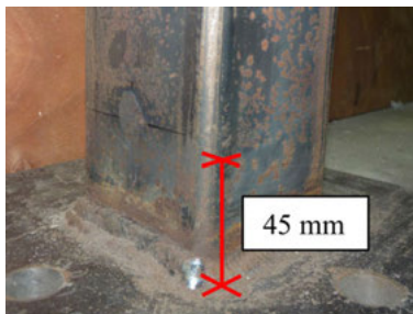
(c) Deformation of SHS-20 (left face)
