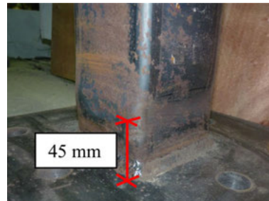
(b) Deformation of SHS-0 (right face)
