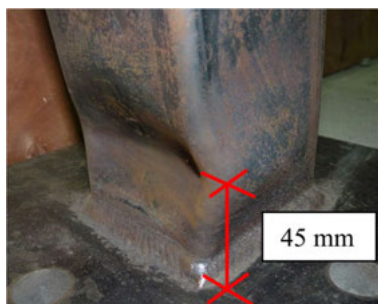
(a) Deformation of SHS-0
