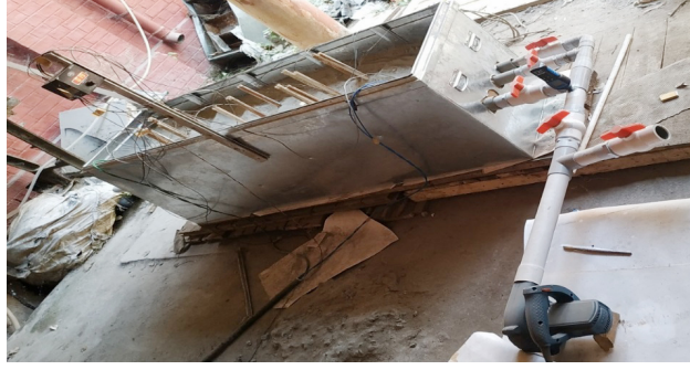
Figure 2: Photograph of the EAHE test rig.
