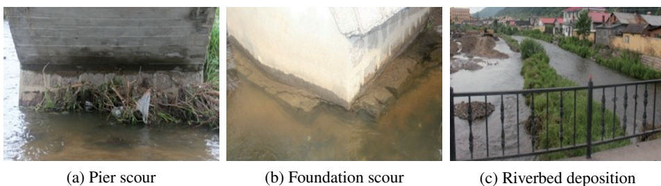
Fig. 4. Main damages of substructure
