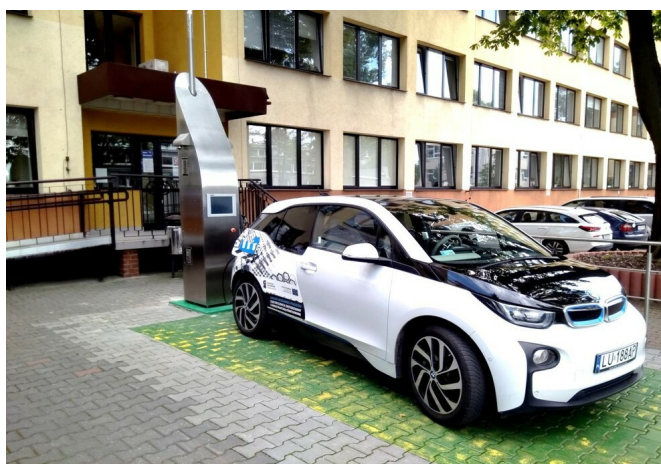
Fig. 1. View of electric vehicle charging station under study
