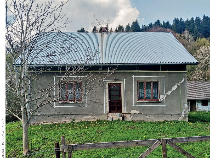
Cracks forming in the walls of a residential building built on landslide colluvium – Dąbrowka Starzeńska, Dynów municipality
