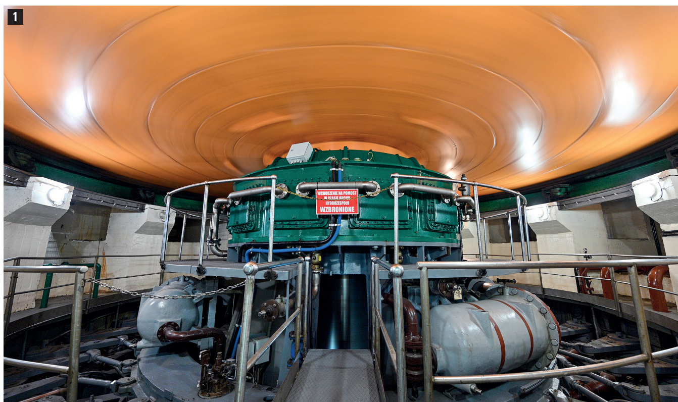
Photo 1 A working hydropower unit (showing the support bearings and generator rotor)
