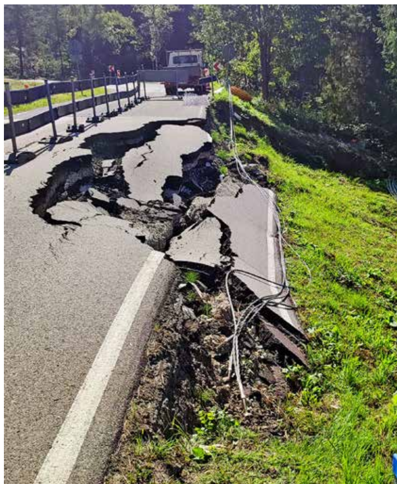
Landslide-damaged fragment of road between Wetlina and Brzegi Górne
