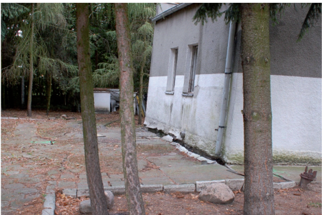
Visible inclination of the building by about 25 cm towards the river in the closed wastewater treatment station of the Correctional Facility in Wronki
