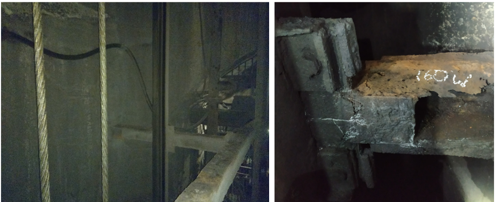
Fig. 3. Corrosion in a mine shaft
