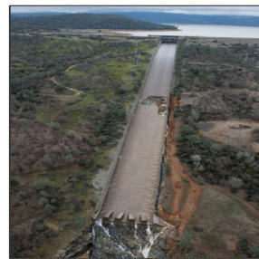
Oroville Dam incident: Concrete spillway
