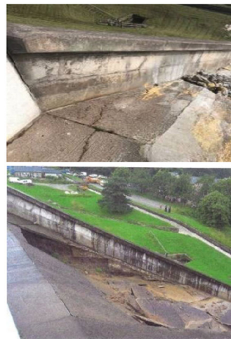
Toddbrok Dam incident: Shallow foundation and spillway cracking
