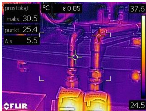
Fig. 4. Thermographic investigation of the cooling sub-system.
