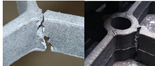
Fig. 2. Cracks formed in grate wall connections
