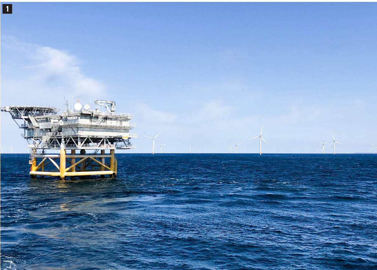
Photo 1 A platform with an offshore transformer station at the Anholt wind farm in Denmark
