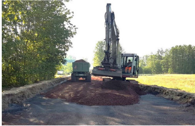
Fig. 8. Realization of the reinforcing layers of aggregate reinforced with a geogrid (section II)
