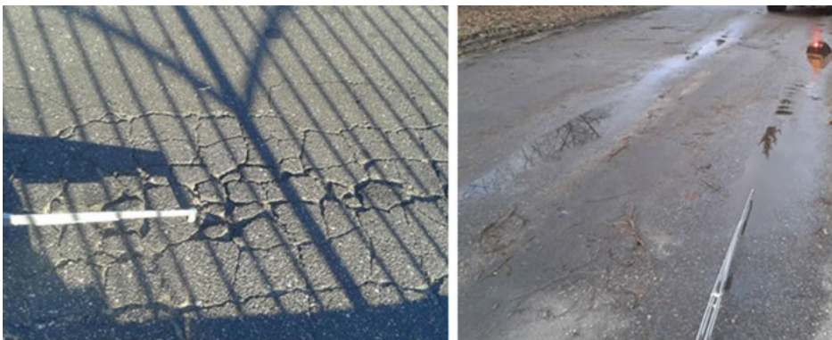
Fig. 2. Typical road damages, left – mesh cracks, right – longitudinal ruts
