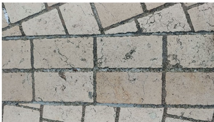
Fig. 8. Damages of Hauteville limestone paving stones in Mariacki Square in Krakow
