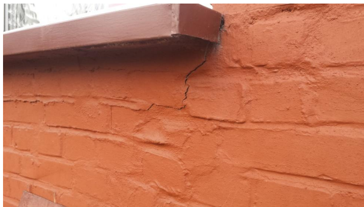
Fig. 19. Crack in the corner of the window opening of building #3 (Source: own study)
