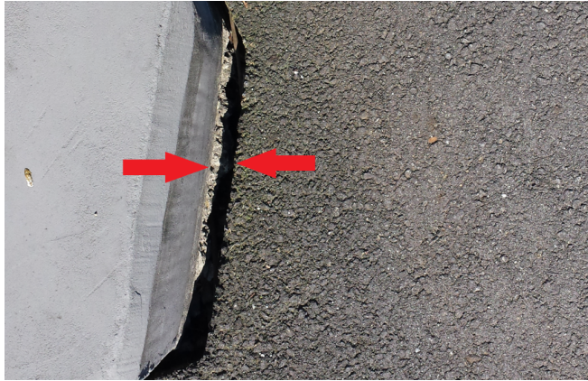
Fig. 8. Detachment of the asphalt surface from building no. 1 (Fig. 7) (Source: own study)
