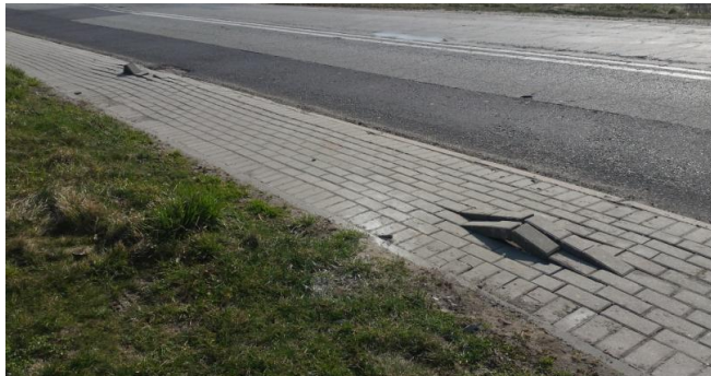
Fig. 9. The uplift of paving stones (location – blue circle, Fig. 7) (Source: own study)
