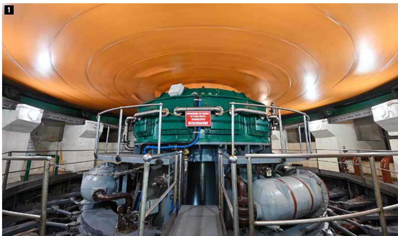
1 Photo 1 A working hydropower unit (showing the support bearings and generator rotor)
