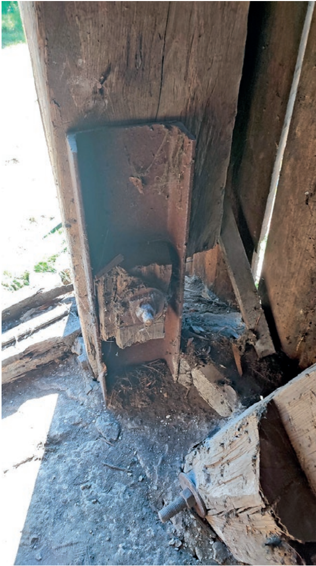
III. 11. The existing condition of the lower sections of the posts indicates that no joint replacement was carried out. Measures were limited to cutting off the lower parts of the posts and setting new foundations with joints using vertical channels. Source: original photo, 2023
