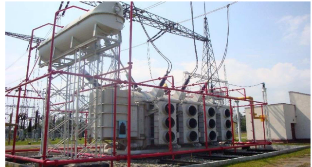
Fig. 1. General view of the tested transformer at the work station.
