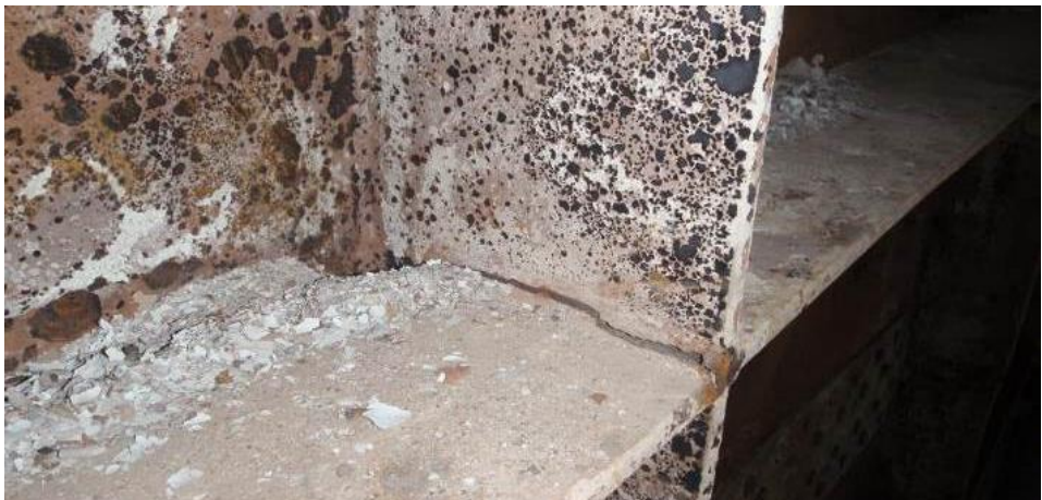
Fig. 9. Typical crack of weld
