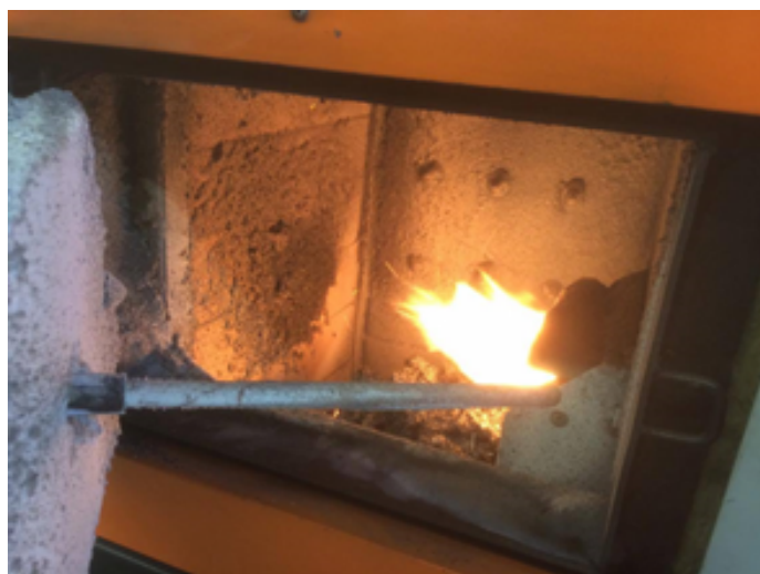
Fig. 5. Thermocouple's position in the boiler combustion chamber
