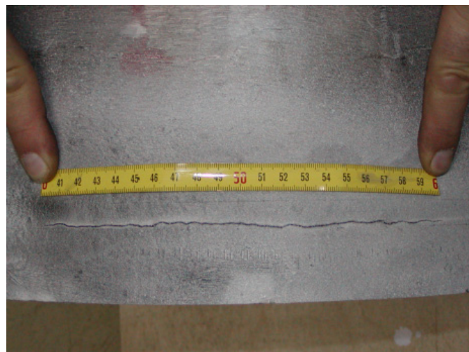
Fig. 1. The main crack - a view from the outer side in the place of the welded joint
