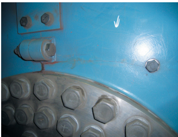
Fig. 1. Side disc cracks above the hub
