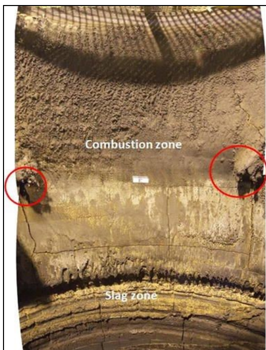
Fig. 3. View of the combustion and slag zone at the eastern furnace side. Severe corrosion of the refractory in the slag zone. Formation of massive build ups at the lance ports (circles) [9]
