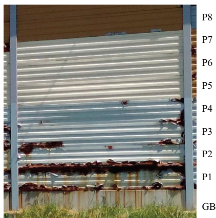
Fig. 17. Corroded acoustic screen
