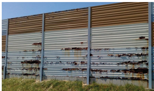
Fig. 1. Corroded acoustic screens on the expressway S11 in Skrzyńki (Poland) next to Kórnik-North junction
