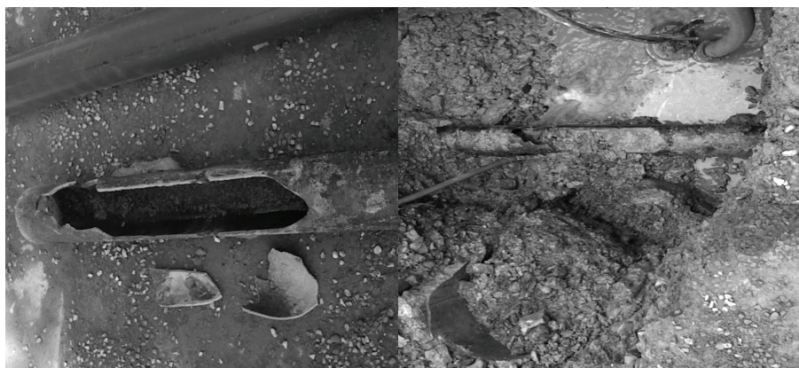
Fig. 1. The example of influence of soil properties to corrosion of water pipe (own study)
