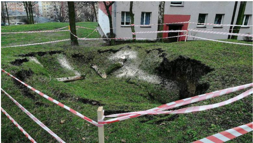
Fig. 3. Sinkhole in the former mine field of “Jan Kanty”, Jaworzno GZW Poland (Polska Times, 2017)
