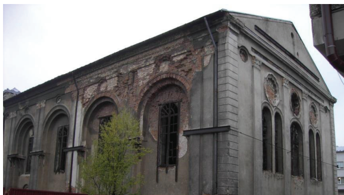
Fig. 4. Synagogue in Dąbrowa Tarnowska. Southern elevation. Damage to the wall caused by rain water.
