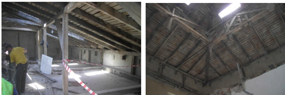
Fig. 13. Building of Cracow University of Economics. Roof structure before and after rebuilding.
