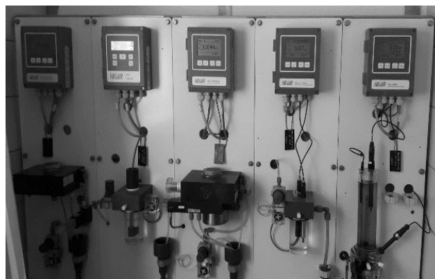
Photo 1. Automatic dosage and monitoring of chlorine concentration in water for disinfection and monitoring the kinetics of water reactions (phot. V. Beluli)
