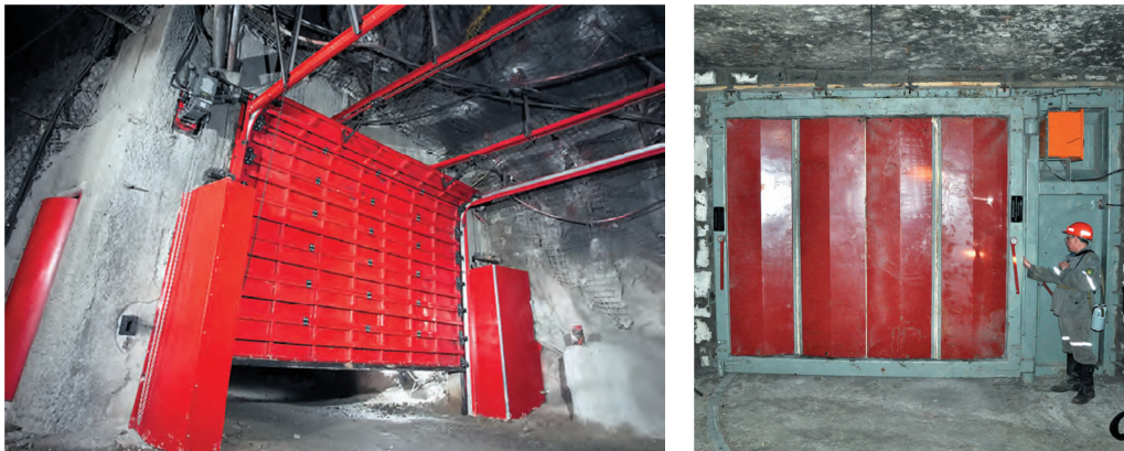
Fig. 5. Automated ventilation doors: vertical lift of the leaf (left), turning louvers (right)
