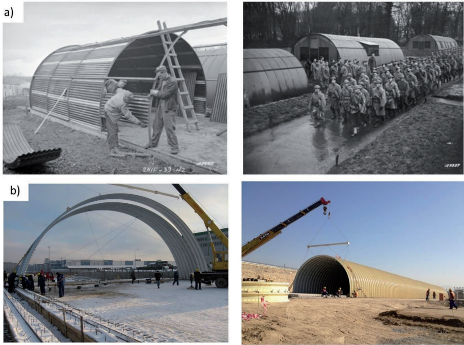
Fig. 1. Double corrugated arch structure facilities, a) historical photo presenting the Quonset Hut system facility mounting [1], b) K-span system roof structure assembly [6]
