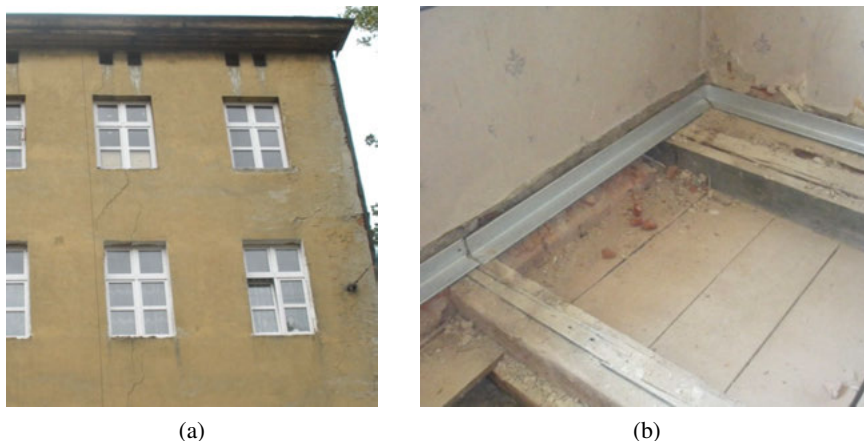
Fig. 8. Tenement house in Łódź, Żeromskiego street: a) cracks on elevation and b) steel bond beam
