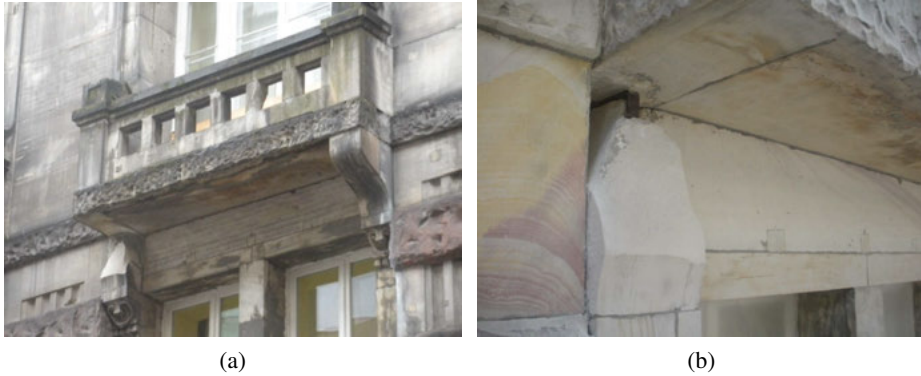
Fig. 11. Warsaw, Kredytowa street 3: a) stone balcony and b) bracket fallen down from the facade
