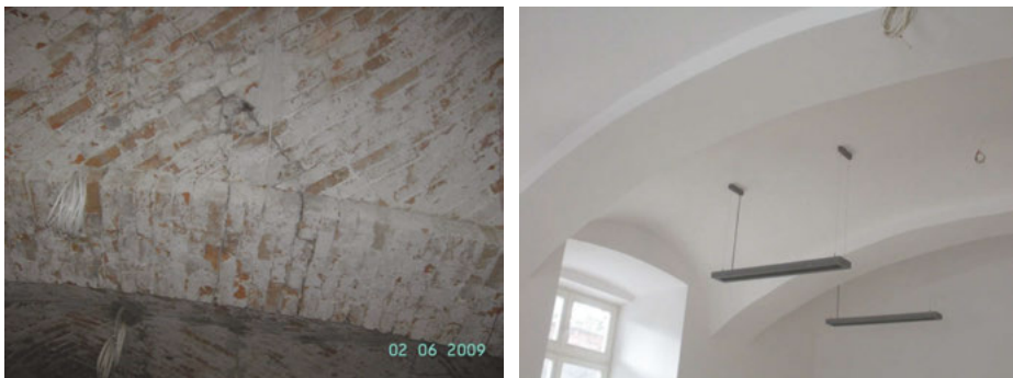
Fig. 6. Royal Palace in Łobzów, Cracow. The vault before (left) and after (right) renovation
