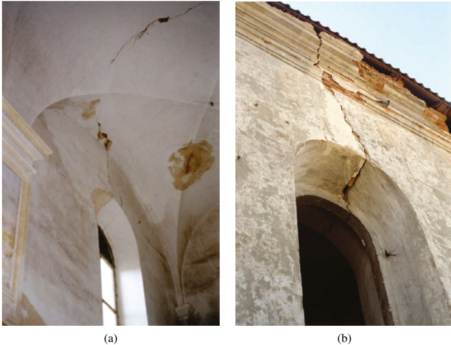
Fig. 9. Synagogue in Słonim, Belarus: a) cracks of the vault and b) the arch above window
