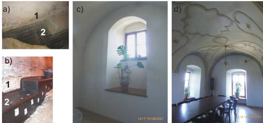
Fig. 8. South-east corner of the east wing in the Dominican monastery: a) and b) the micropiled structure supporting the corner – the internal and external grid beams photographed under construction (1 – east wall, 2 – micropiled structure), c) present view of the restored corner room in the ground floor (the wall shown in Fig. 3b), d) present view of the restored corner room in the first floor
