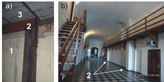
Fig. 9. Steel structures unloading the vaults in the east wing of the Dominican monastery founded on the transverse first floor wall: a) one of steel frames under construction, b) present view of the corridor in the second floor lined with the steel frame (1 – longitudinal wall standing on the vault, 2 – steel frame, 3 – ceiling above the second floor)
