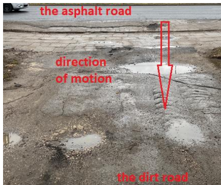
Fig. 2. The place of the analyzed traffic issue on the dirt road after leaving the asphalt road
