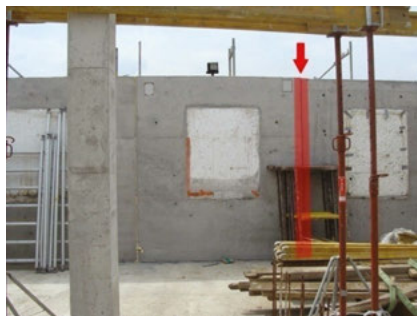
Fig. 8. Reinforced concrete column location in the building erected in the POLYTECH system
