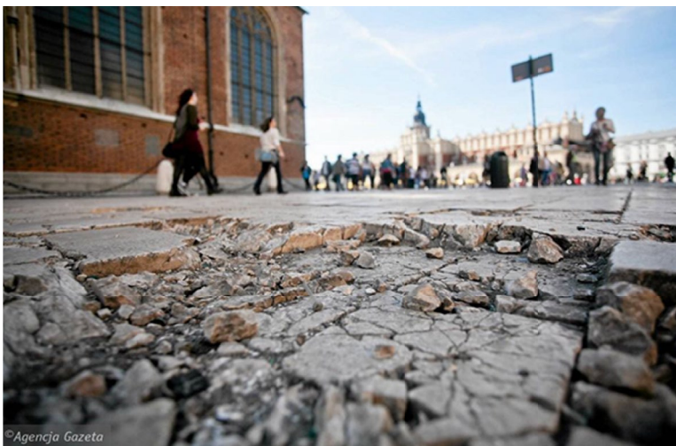
Fig. 4. Numerous cracks and damages of Turkish limestone paving stones [15]
