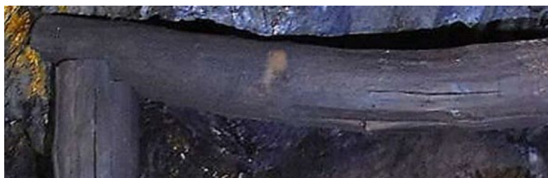
Fig. 2. Damaged prop and roof-bar (enlarged photograph from Fig. 1)
