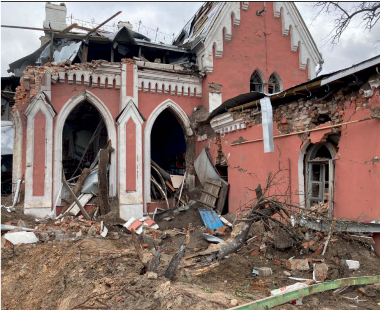
Ill. 7. The damaged Vasyl Tarnovsky's mansion in Chernihiv. Photo by A. Glushchenko (director of the Department of Urbanism and Architecture of the Chernihiv Regional State Administration).
