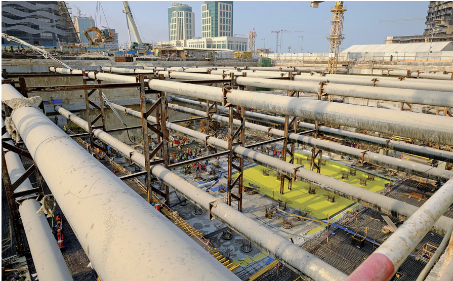
Fig. 1. An example of a commonly used approach for implementing the underground part of a project based on the use of steel struts [14]
