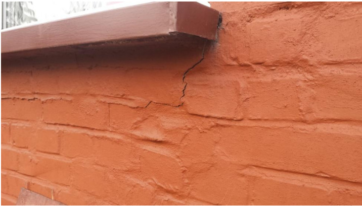
Fig. 19. Crack in the corner of the window opening of building #3 (Source: own study)
