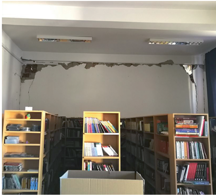
Fig. 8. Detachments at the joint of the infill wall and the reinforced concrete frame and damage to the wall corners (school in Petrinja after the earthquake in December 2020)
