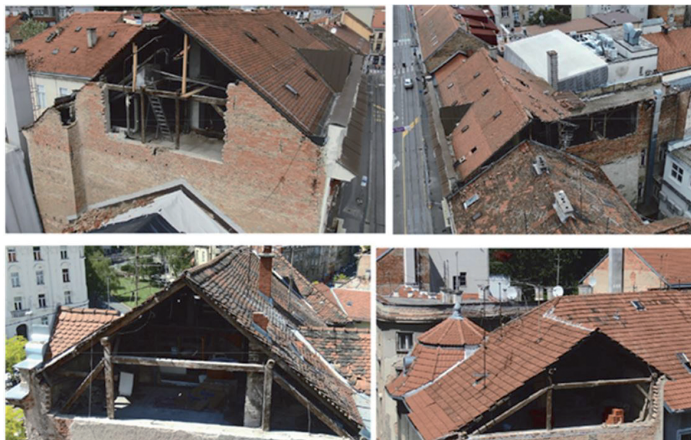
Fig. 4. Destroyed out-of-plane gable walls after the Zagreb earthquake (March 2020), caused by the impacts of wooden roof truss elements [12]
