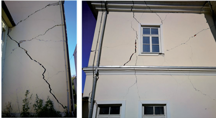
Fig. 2. Wall damage (in-plane) in the center of Petrinja (October 2021)
