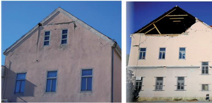
Fig. 3. A closed school building in the center of Petrinja with out-of-plane gable damage (October 2021)
