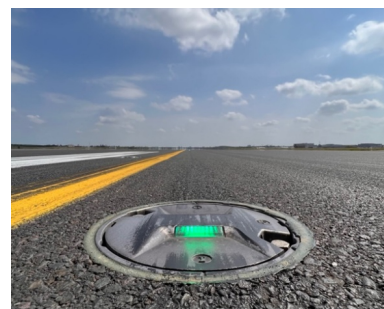
Fig. 1. Airport taxiway centreline in-pavement lamp.
