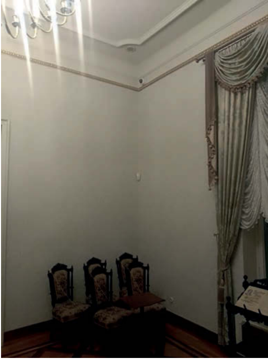
Ill. 5. The same technical devices in historical building of Izrael Poznański Palace in Łódź, Poland, as shown in Ill. 4. Distant view presenting devices with the surrounding. Photo by T. Omieciński, 2023.
