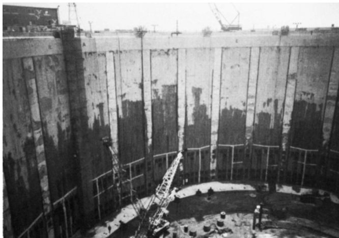
Fig. 2. Cracking of diaphragm wall on Kawasaki Island [7]
