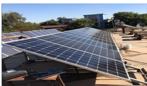
Fig. 1. The solar panels of the system 2 kWp.
