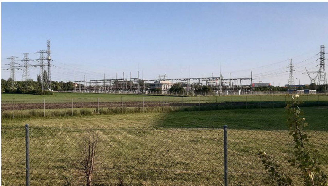
III. 7. Klecina wedge: Transformer station: the Main Power Supply Point "Klecina" R-1. Photo by J. Rubaszek.
