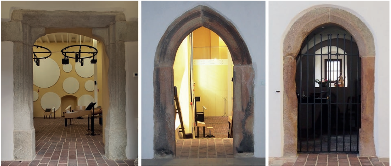
III. 9. Złoty Stok, former Corpus Christi church, portals: a) in the south porch; b) in the lodge; c) in the sacristy. Photo by the Authors.
