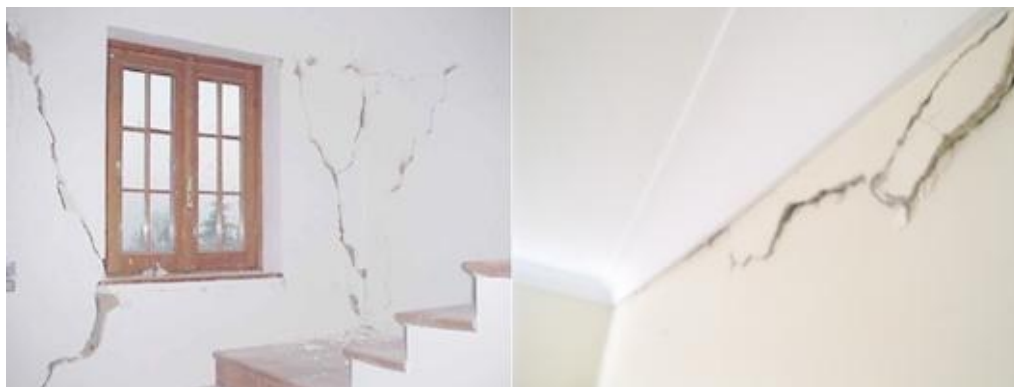
Fig. 1. Examples of structural damage caused by settlement [8]
