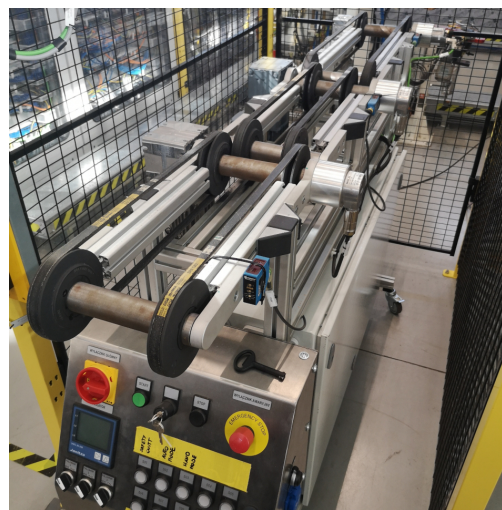
Fig. 1. Belt conveyor controlled by PLC Siemens S7-300
